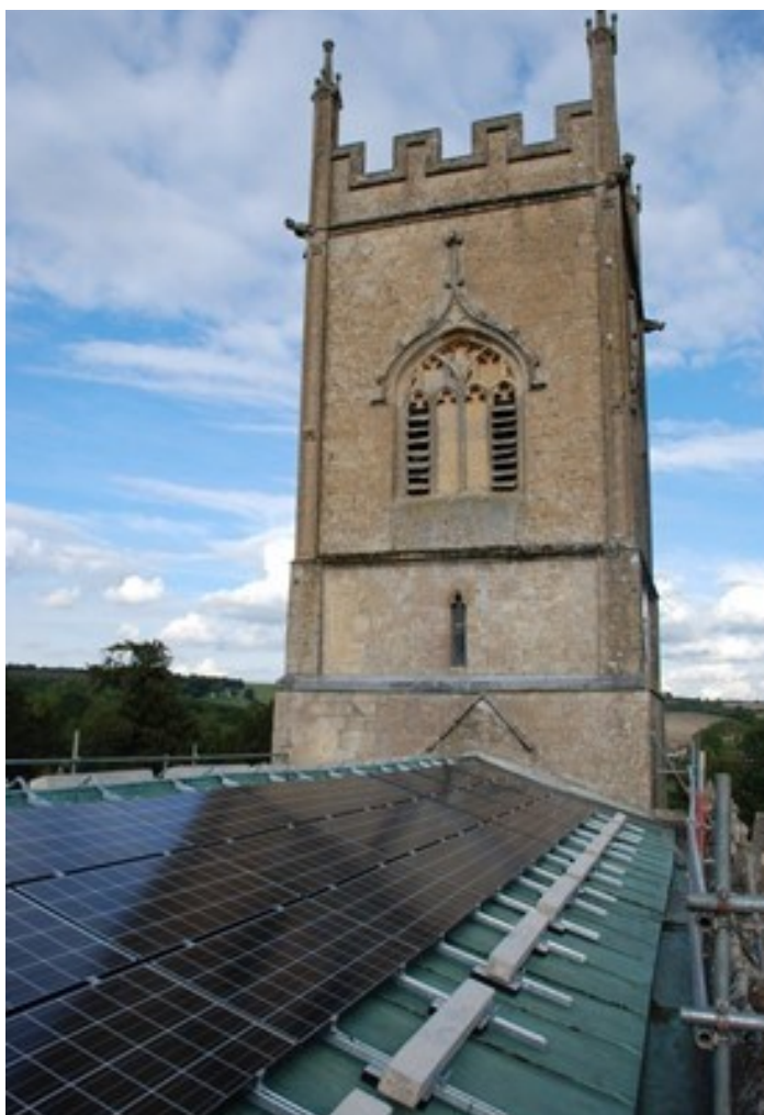
Above: St Michael and All Angel Withington's panels being installed. Read their case study here .
